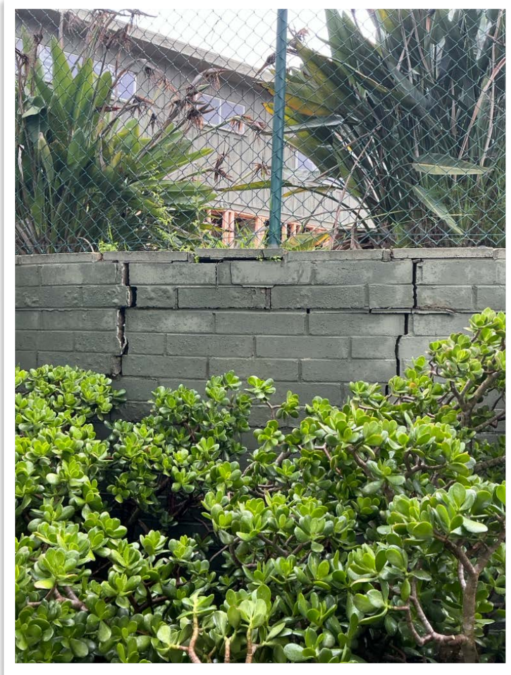
Photo # 8 - There is a damaged retaining wall several feet from the Monterey cypress. In my opinion, this damage is from the soil above pushing it out. Not the tree lifting it. I do not think roots are under the footing.
