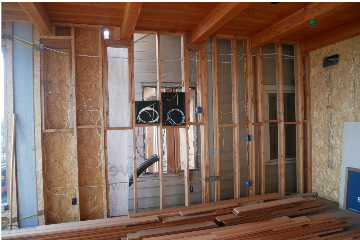
Photograph #22: South elevation at ADU addition added per City of Del Mar approved building permits 8/15/2023
