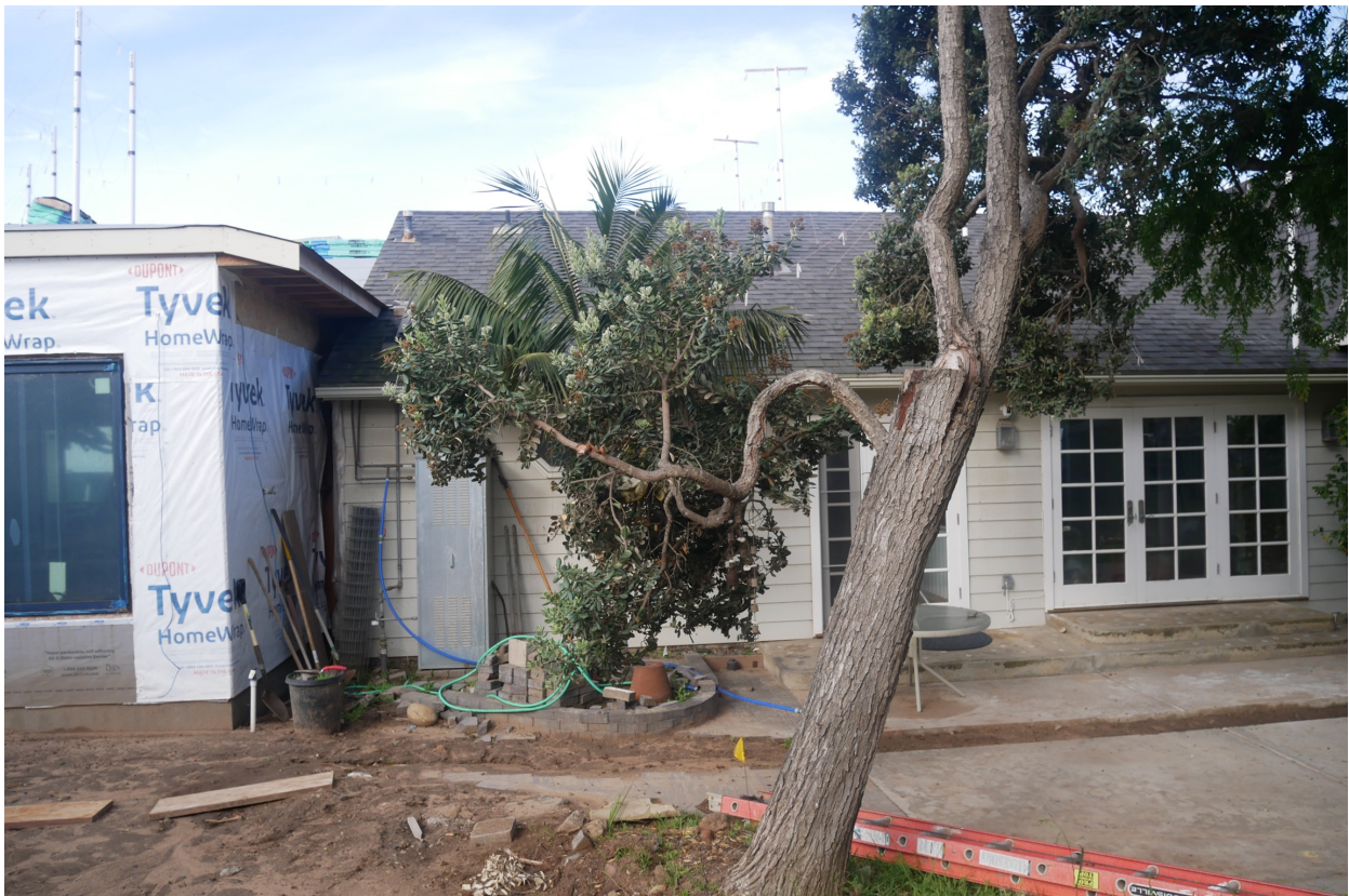
Photograph #17: East Elevation, ground floor porch enclosure added per City of Del Mar Design Review Board Approval 88-64, 2/22/1995 and ADU addition added per City of Del Mar approved building permits 8/15/2023
