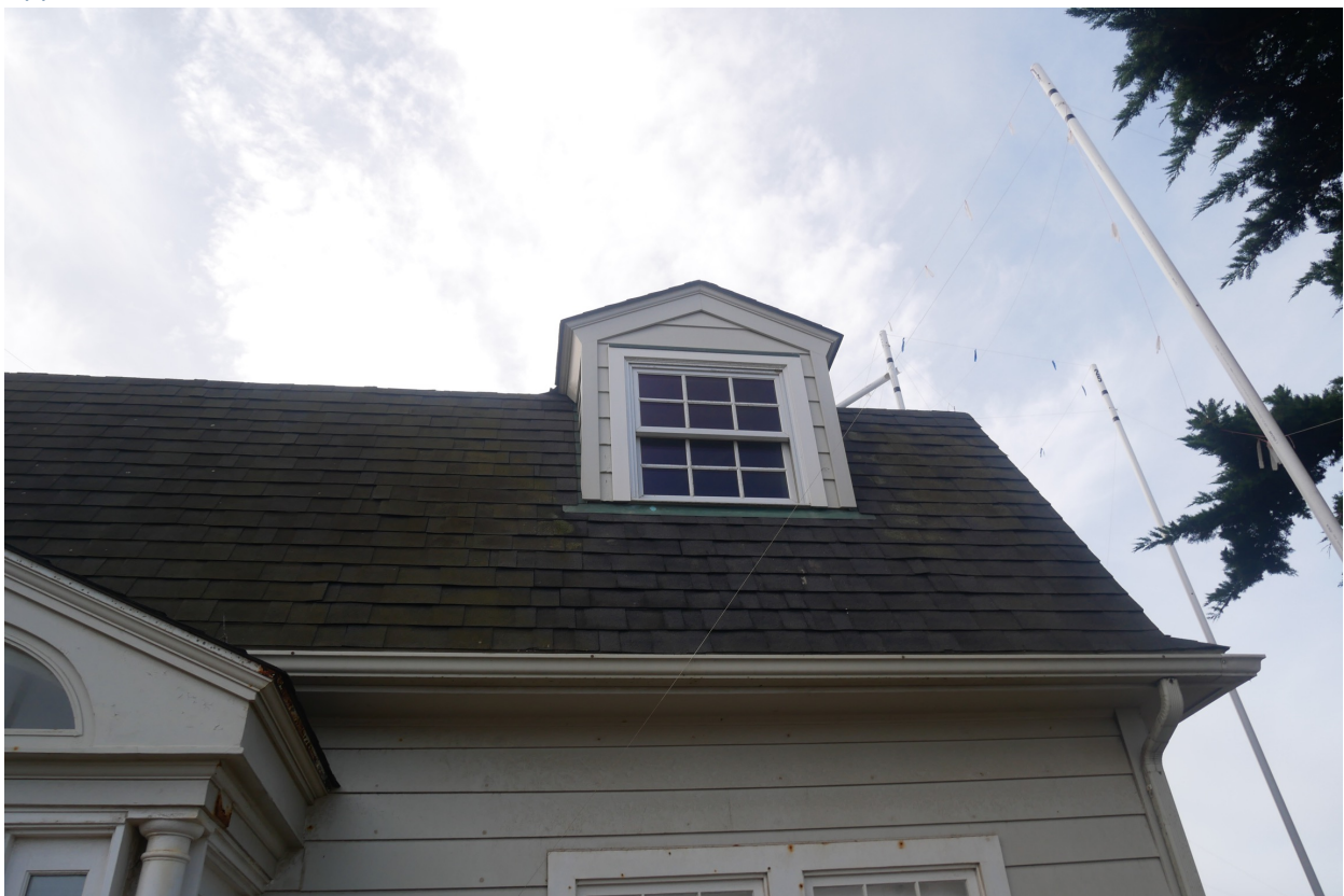
Photograph #9: North Elevation, modified roof dormer window per City of Del Mar Design Review Board Approval 88-64, 2/22/1995
