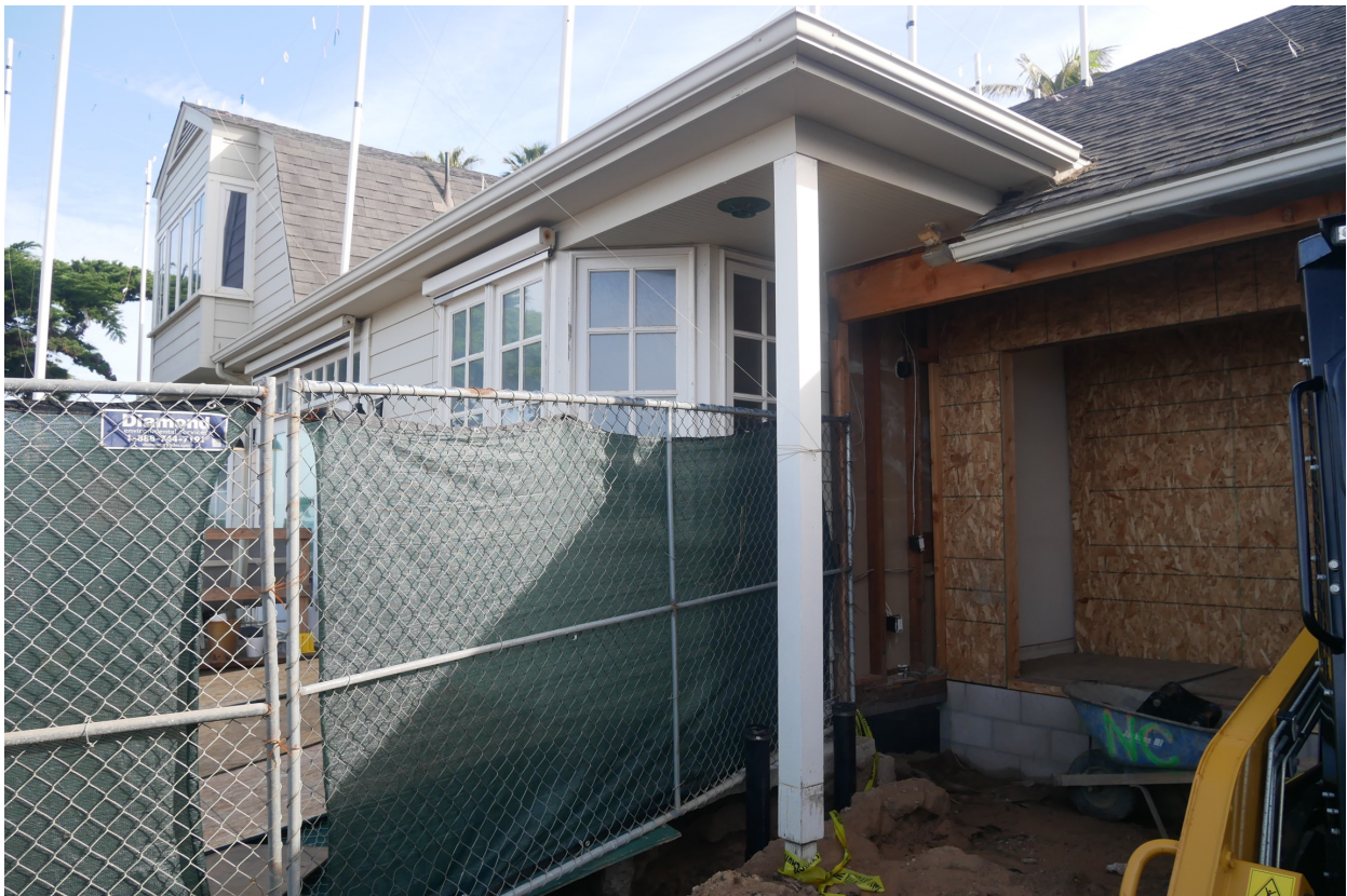
Photograph #24: West Elevation, ground floor porch enclosure added per City of Del Mar Design Review Board Approval 88-64, 2/22/1995 and ADU addition added per City of Del Mar approved building permits 8/15/2023
