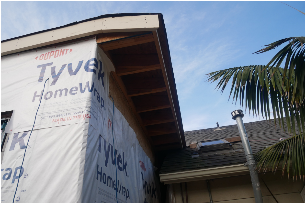
Photograph #21: East elevation ADU addition added per City of Del Mar approved building permits 8/15/2023
