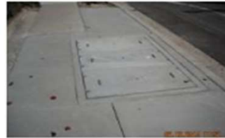
Easement Required for SDG&E Handhole
