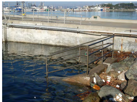
Figure 4.3. Flooded Storm Drain Outfall. 01.20.11, morning : ~7.2 feet above mean low tide.
