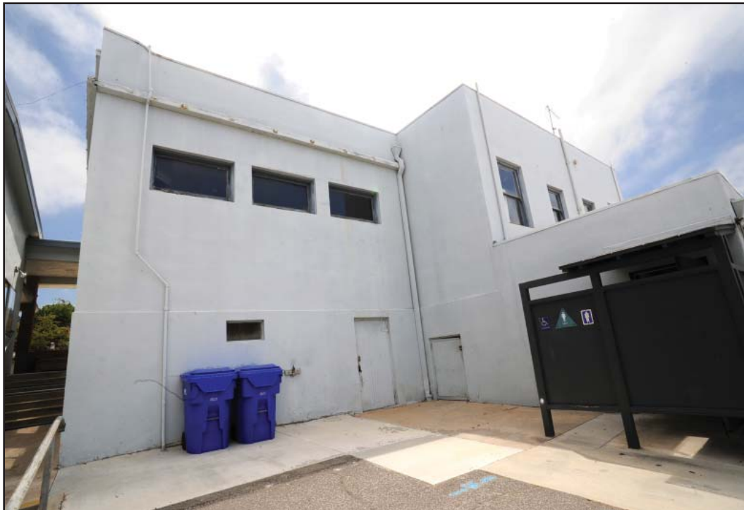
PHOTOGRAPH 8 Building A, North Side of West Wall Showing Bathroom Extension and Small Lip above First Floor Doors
