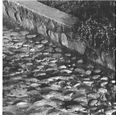
Detail of existing curb and gutter on 12th Street from WPA construction
