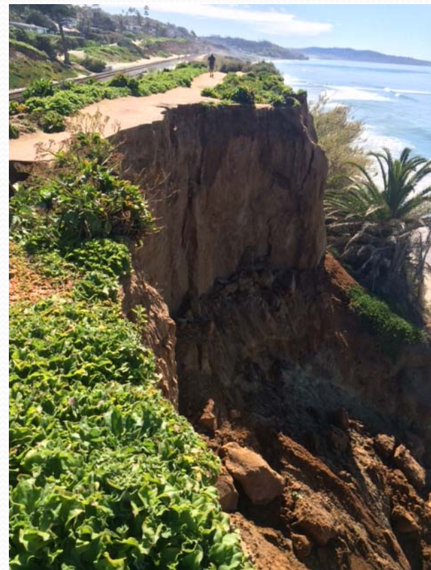
March 2017 Bluff Collapse
