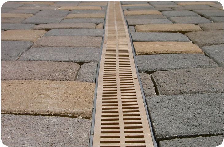
✓ Permeable paving and drains help direct water to on-site storage and percolation.
