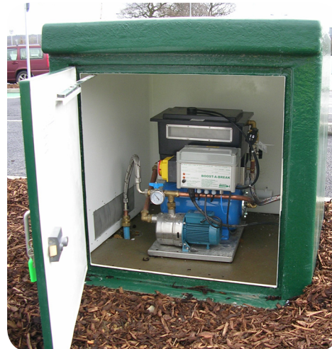
✗ Avoid locating utilities without proper screening.
