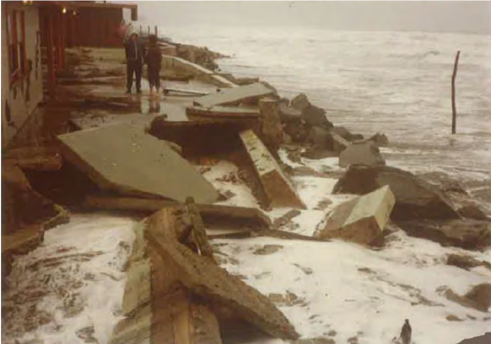
Figure 9.2 Coastal Damage Following 1983 Storm
