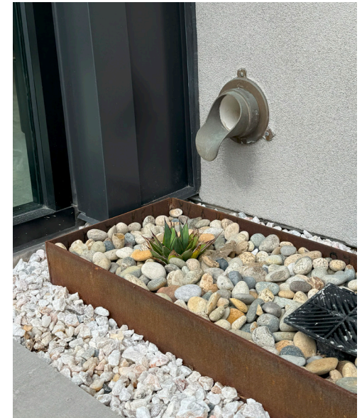
Decorative downspouts feeding plants.
